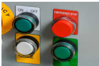
Control panel labels
