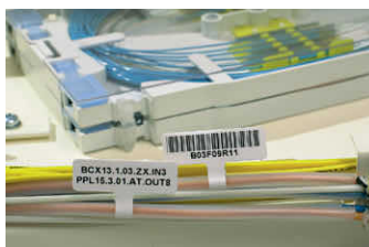
Fibre optic cable markers
